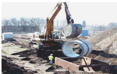
Photo: Cottage Grove Interceptor
